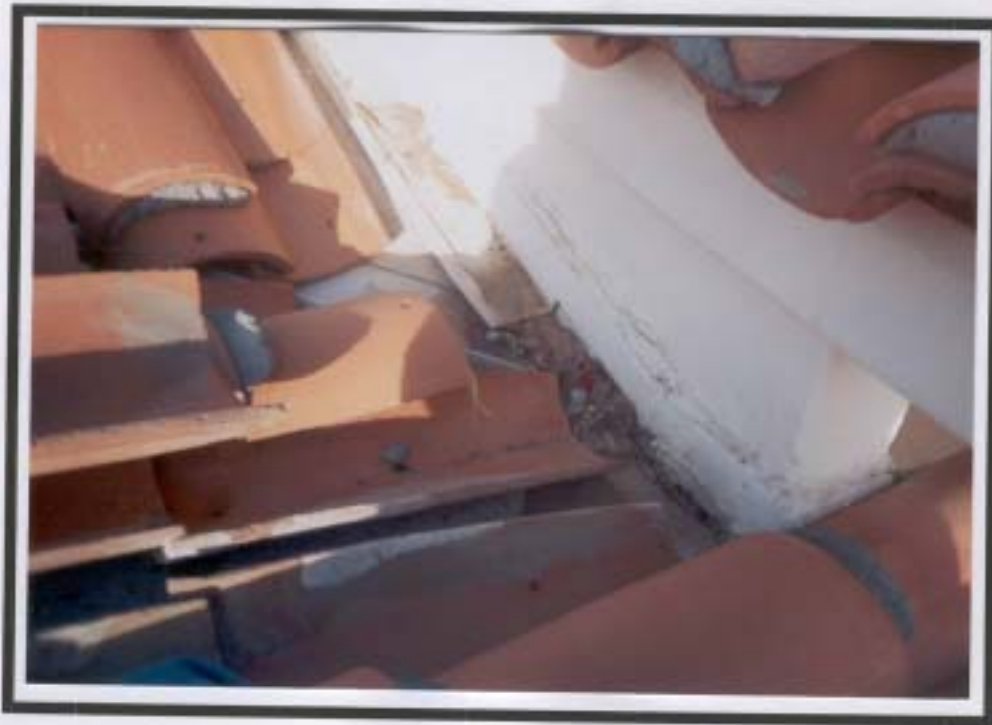
3. Dead valley with tile tops removed. Note inadequate head lap.
