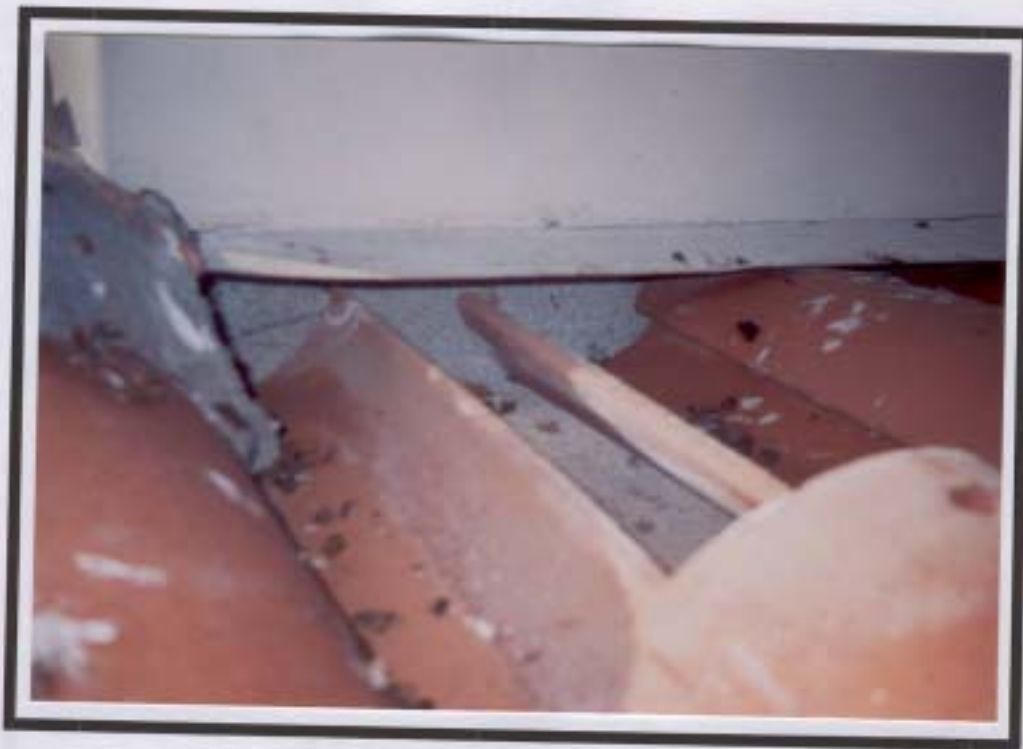
12. Inadequate size counterflashing.
