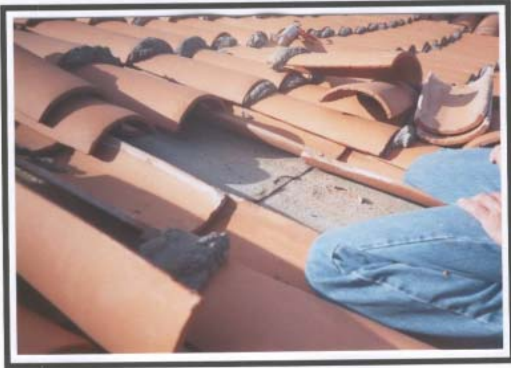
7. Underlayment: Note inadequate head laps and lack of fasteners.
