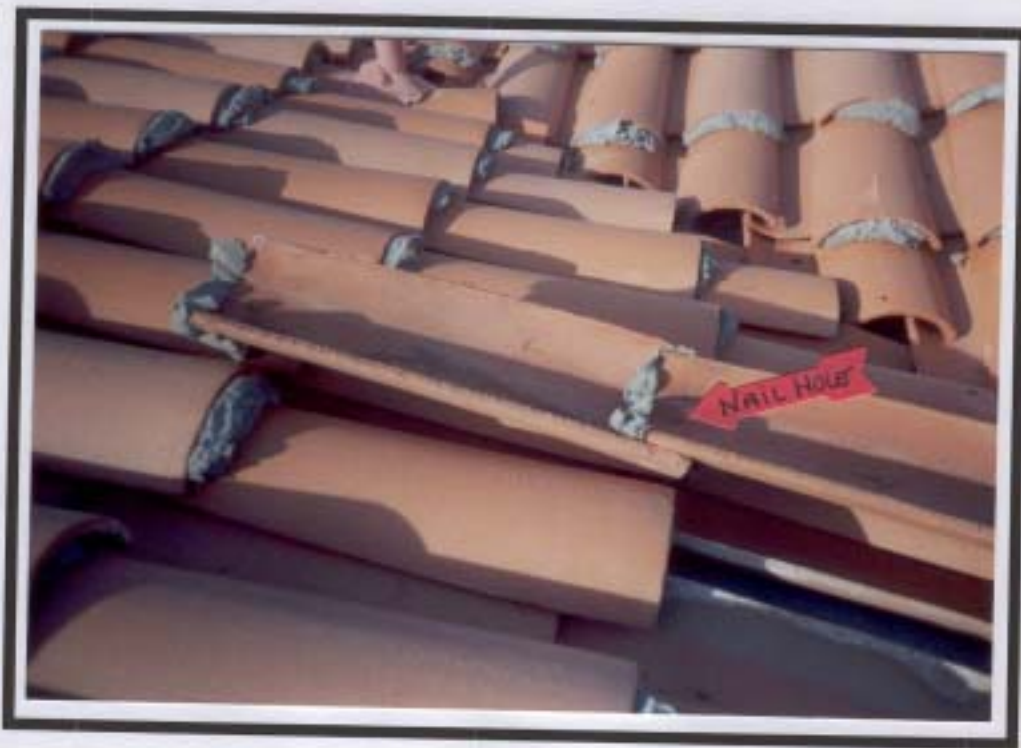
11. Tops have no fasteners and inadequate head lap.
