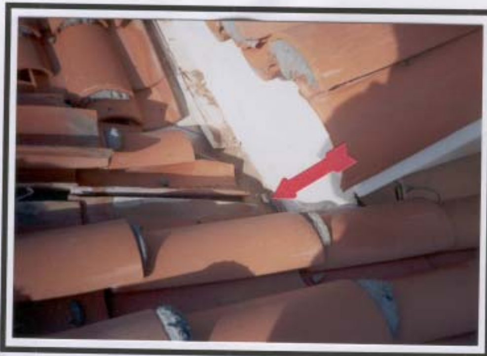
4. Dead valley with debris removed, revealing leak point.
