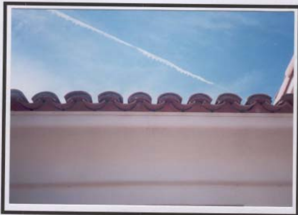
14. View at overhand drip edge.
