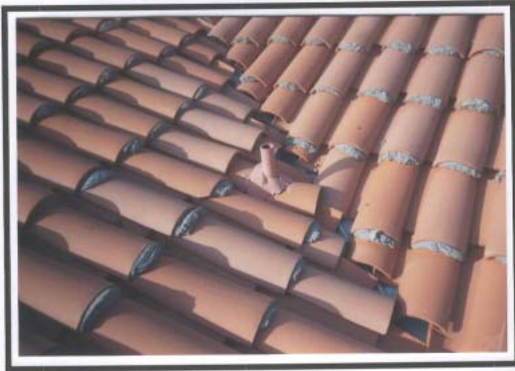
8. Penetration has no lead flashing.
