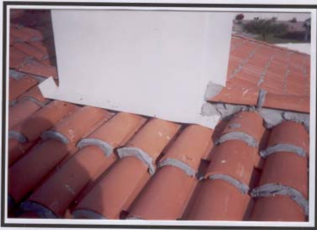
13. Exposed underlayment at chimney with neither metal or mud.
